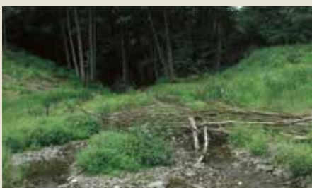
On the Sauerbach stream, once the dam was removed and diggers had dug out the mud, natural watercourse structures soon formed again.
